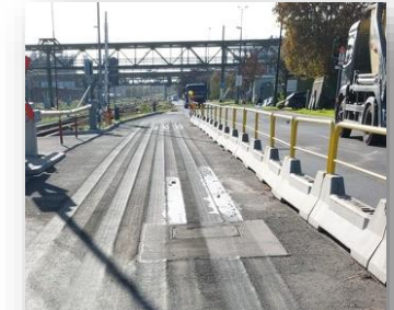
Rutting which will be avoided
